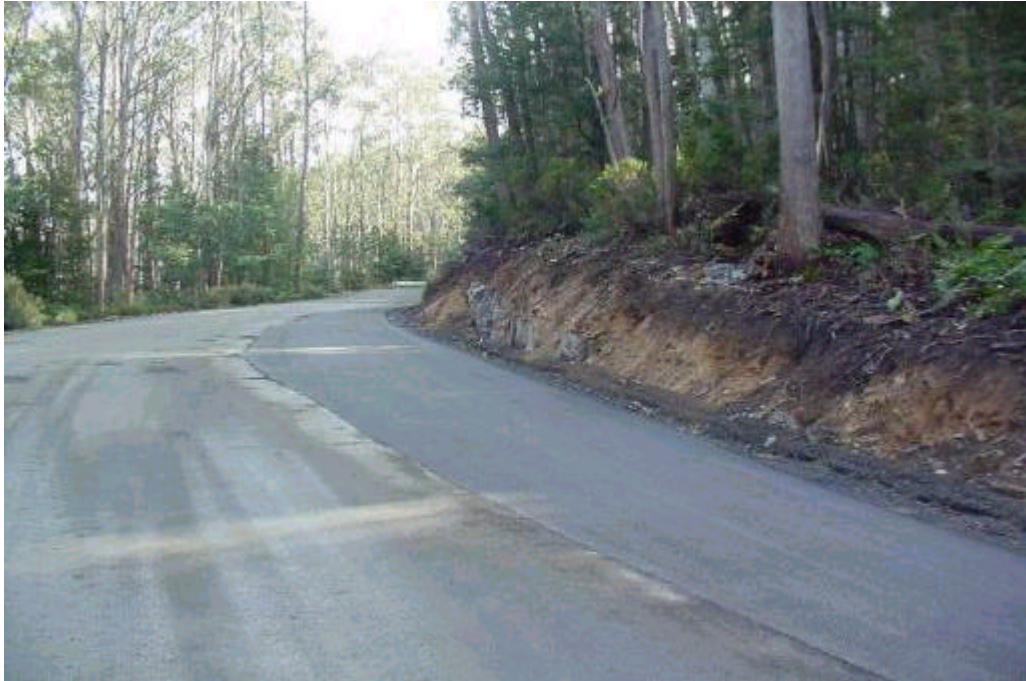
Repaired pavement - Mt Baw Baw access road. (Photo courtesy of the Department of Natural Resources and Environment.) Asset maintenance
