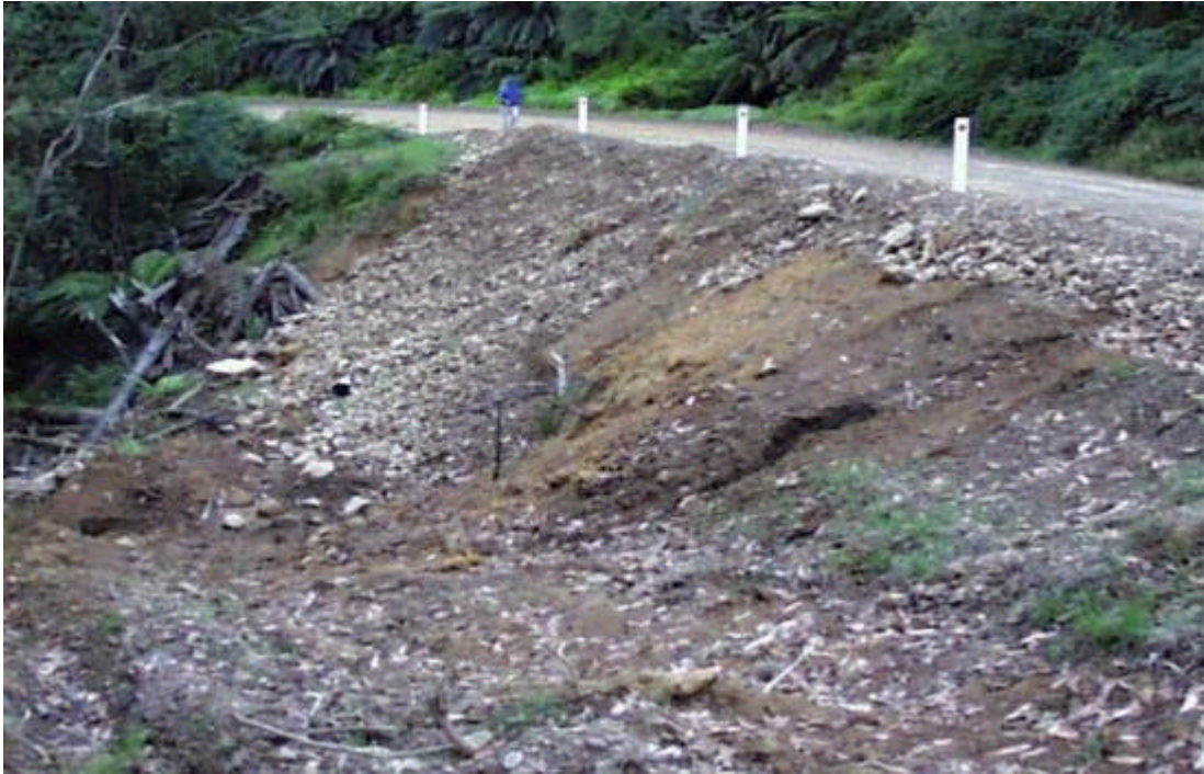
Mt Stirling access road needing repair.
